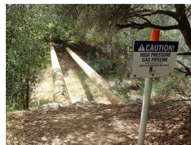
Pipes that service the La Goleta storage field
